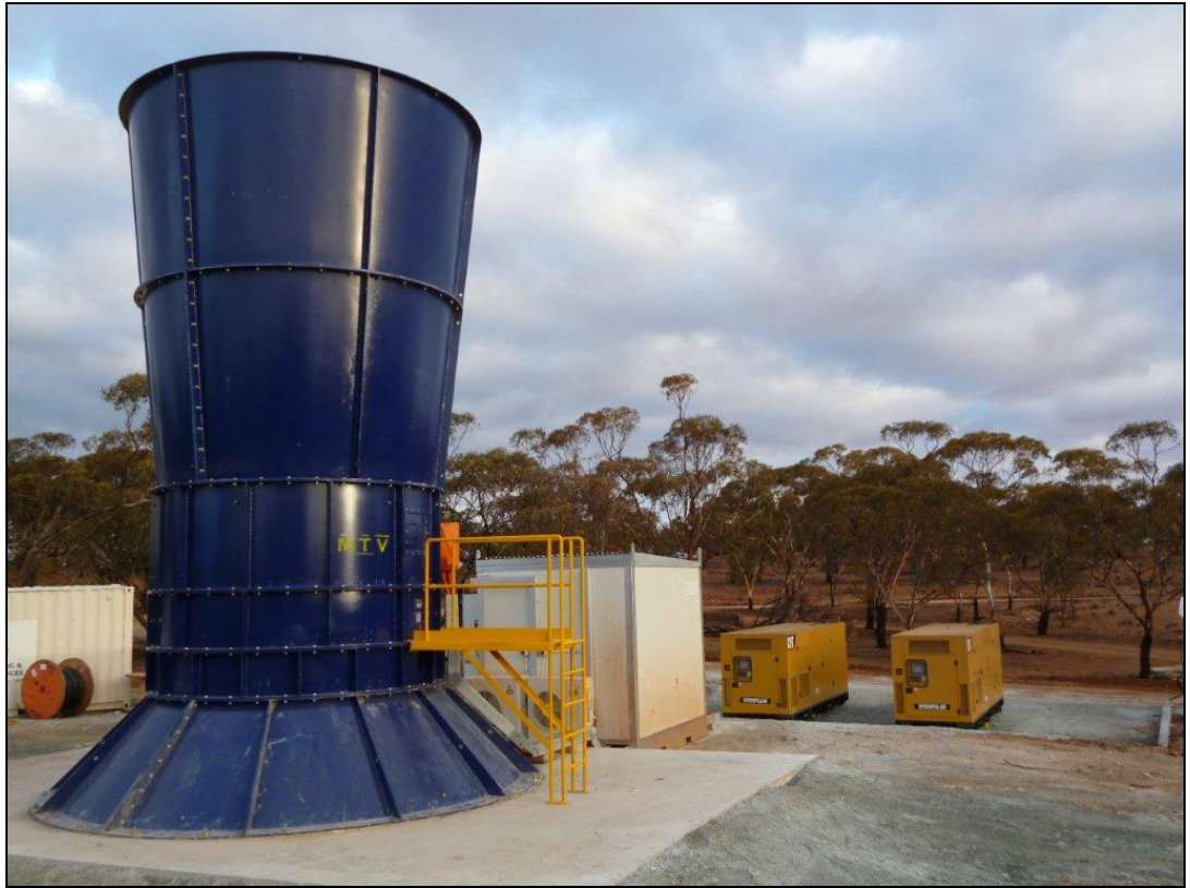
Figure 3: Photo of ventilation shaft collar and primary fan installation.
