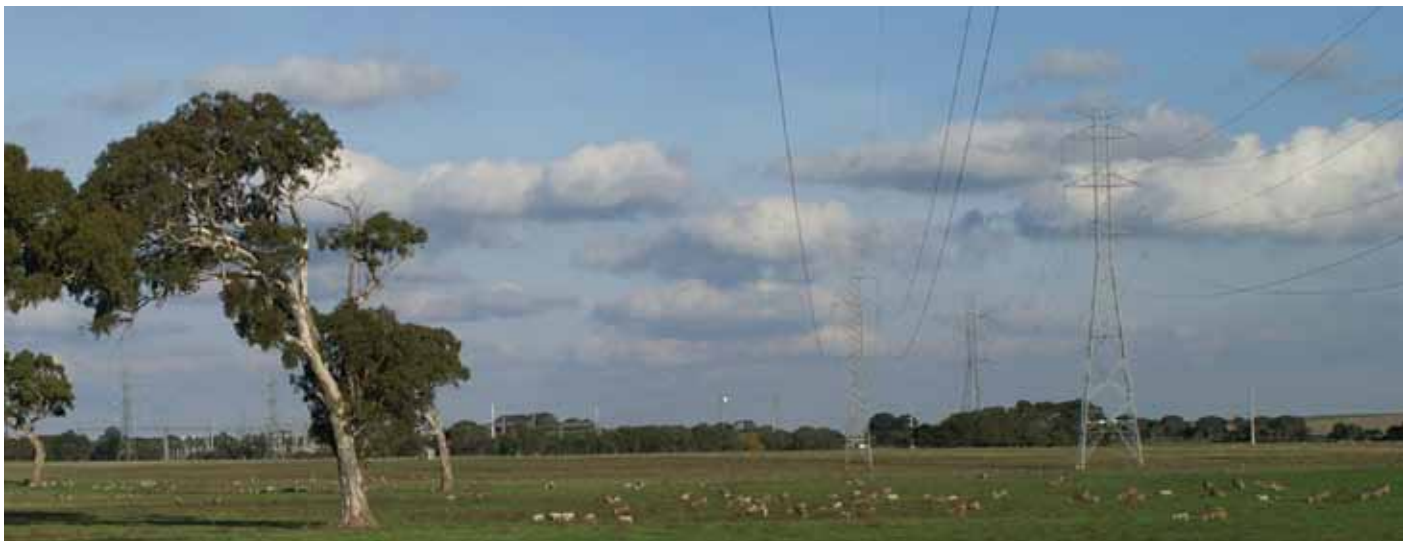
Main power transmission lines crossing Panax's Penola Project Licences.
