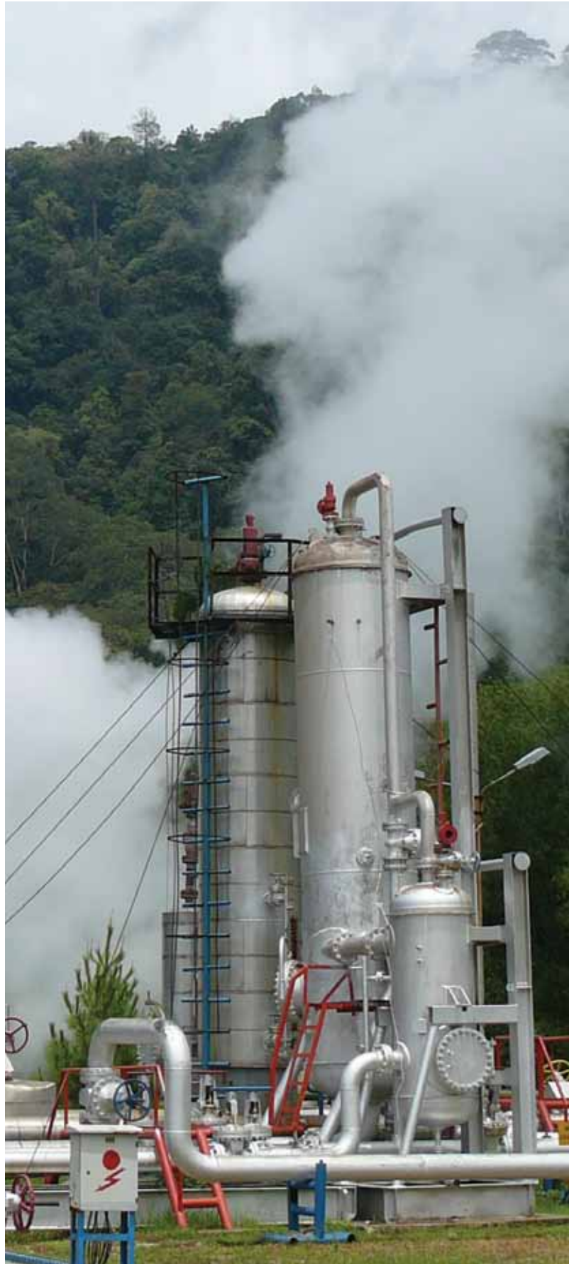
Geothermal plant, northern Sumatra, Indonesia.
