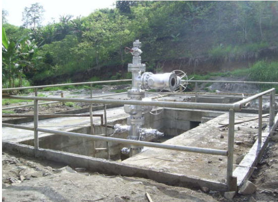
Geothermal well head Sokoria Project, Flores
