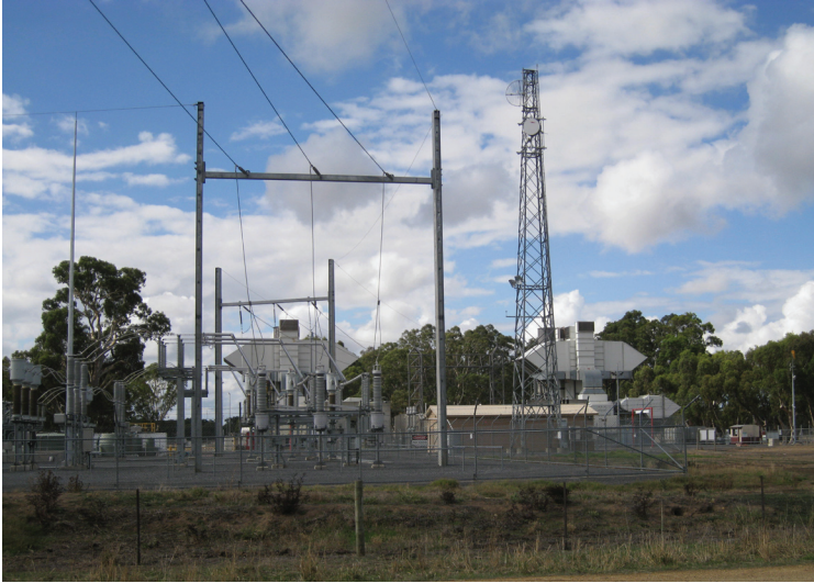
Ladbroke Grove gas fired power station and sub station, Penola region.
