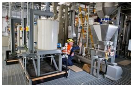
Sulphation and Downstream Facilities - ANSTO
