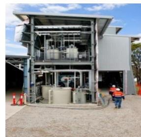
Sulphation section of Demonstration Plant – ANSTO
