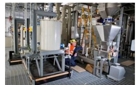
Sulphation and Downstream Facilities - ANSTO
